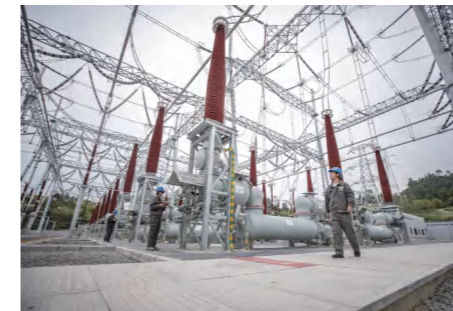
Electric power system
