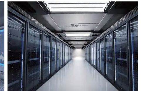
IDC engine room
